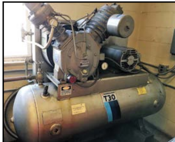
INGERSOLL-RAND 10 HP AIR COMPRESSOR
