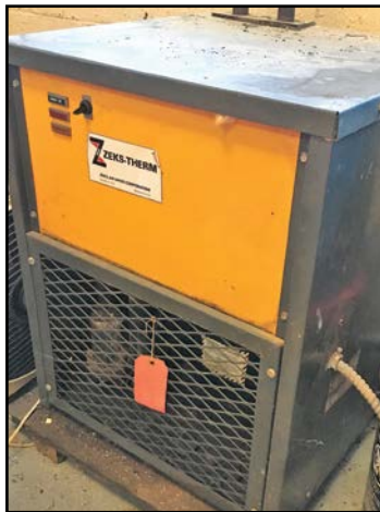
VIEW of ZEKs AIR DRYER
