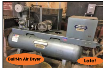
SAYLOR-BEALL 5 HP AIR COMPRESSOR
