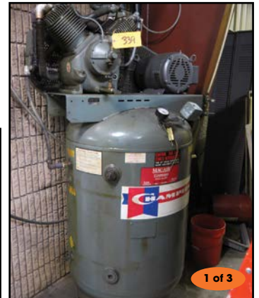
VIEW OF AIR COMPRESSOR
