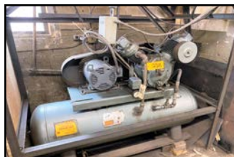
INGERSOLL-RAND 7.5 HP AIR COMPRESSOR
