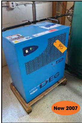
MTA # DEG-0075 "REFRIGERATED" AIR DRYER
