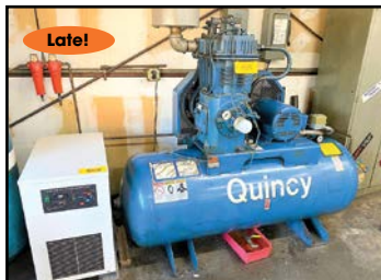
VIEW of QUINCY AIR COMPRESSOR & AIR DRYER
