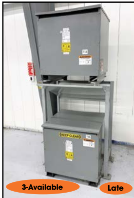
3-Available Late VIEW of 75KVA TRANSFORMERS
